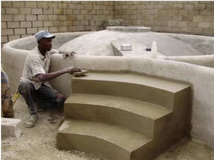
Figure 6 biodigester à Kaynou, Belair
